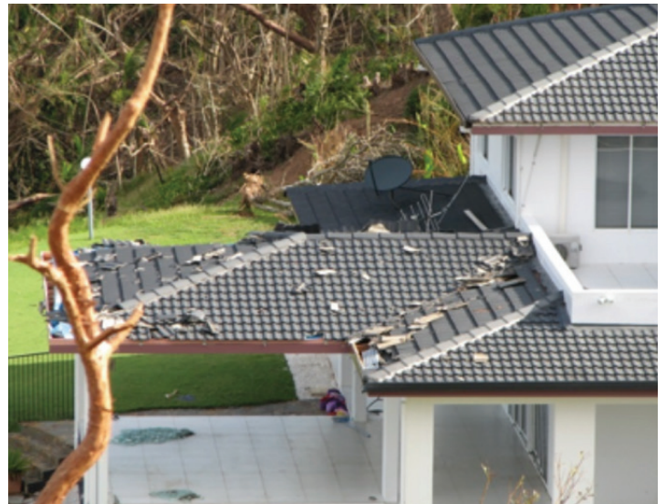
Photograph 3 - Inadequately fixed tiles dislodged after high wind event
