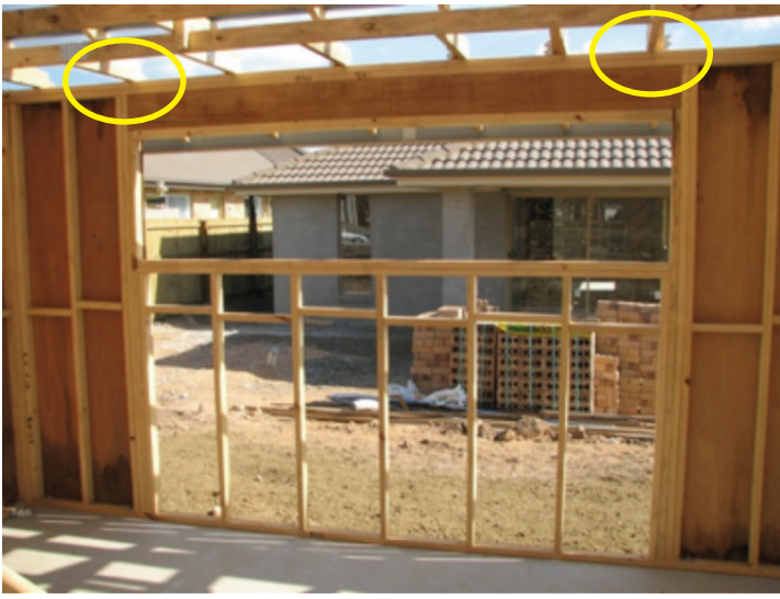
Photograph 11 – Plywood cannot be used to effect tie-down at sides of openings as the trusses highlighted above must have 300 mm min of ply to the right and left side respectively
