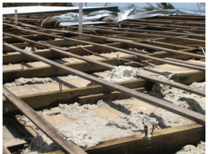
Photograph 4 – Roof sheeting 'blown' off due to inadequate fixing of the sheeting to the battens
