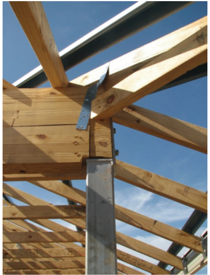
Photograph 16 – Intersecting verandah beams. The LH beam has inadequate bearing and tie-down capacity
