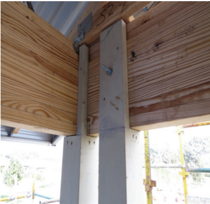
Photograph 14 – Posts over checked, bolted connection would not achieve any tie-down capacity
