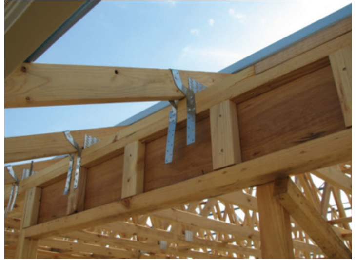
Photograph 9 – Incorrect practice for tying down over openings as top plates not tied to lintel
