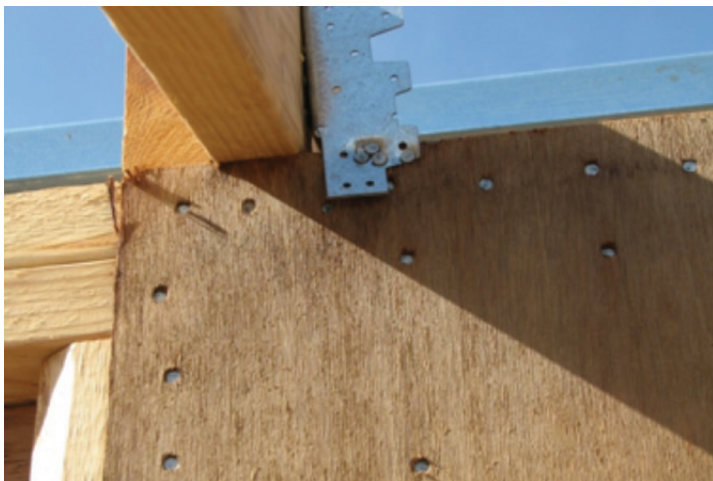
Photograph 2 - A structurally inadequate and incorrectly installed multi-grip. Nails too close to each other and edge of metal and also, too close to top edge of top plate
