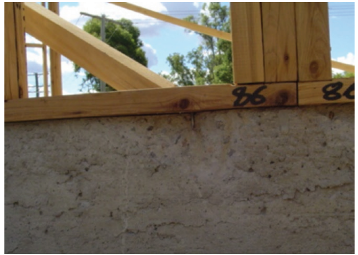
Photograph 13 – Nominal bottom plate connection compromised by excessive plate overhang
