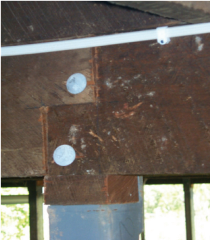
Photograph 15 – Minimum bolt end distances less than required to achieve uplift capacity. Also, unseasoned timber packer used is not suitable due to shrinkage
