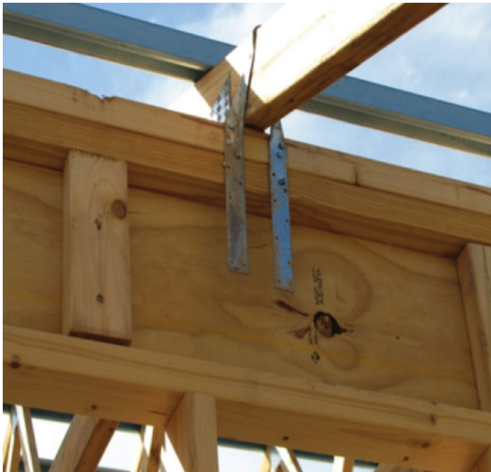
Photograph 1 - Inappropriate practices as nails are too close to strap edge, too close to pre-punched holes and even doubled up. Strap should also have been installed on the inside of frame to enable strap nailing direct to lintel without bending the strap
