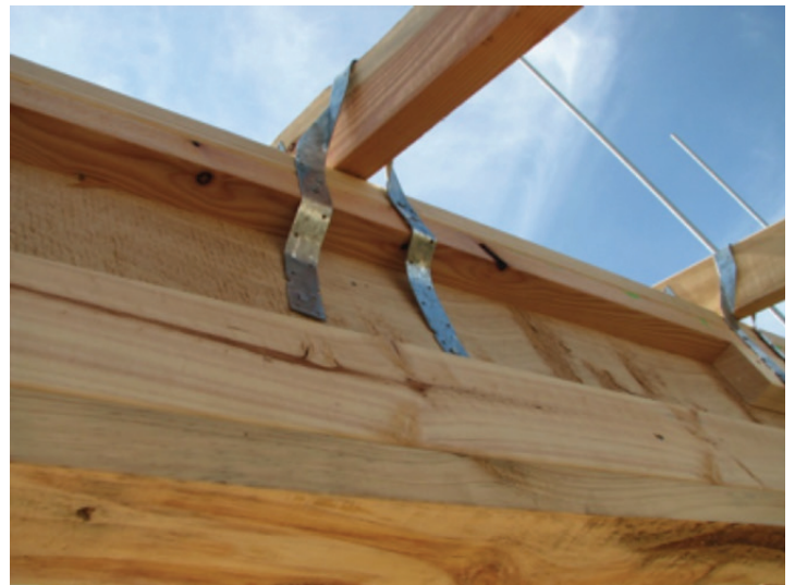
Photograph 10 – Truss tied direct to top plate and lintel, but strap bent through too great an angle to be effective
