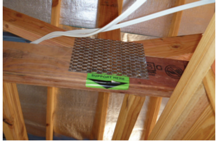
Photograph 6 – Girder truss incorrectly supported by an offset wall
